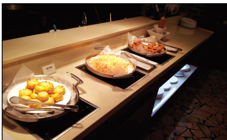
Multiple DWR04's installed with stainless steel trim in buffet counter
